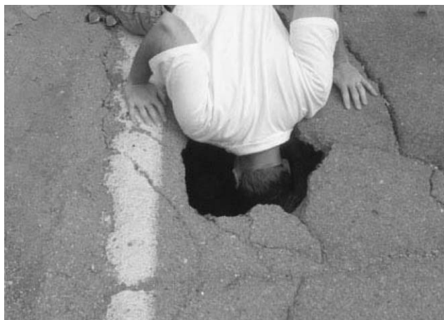
Fig. 3 The middle of Samuelson Road in Portage, Ind., has a pothole the size of a person's head. © American Consulting Inc. Photo by Sean Porter; http://www.asce.org/reportcard/2005/assets/gallery/2-head.jpg .
