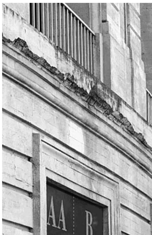
Fig. 1 Crumbling façade of the Memorial Stadium at the University of California, Berkeley. Photo courtesy of Liz Mangelsdorf, San Francisco Chronicle, 2004; http://www.sfgate.com/c/pictures/2004/09/09/sp_calstadiumfacade.jpg .
