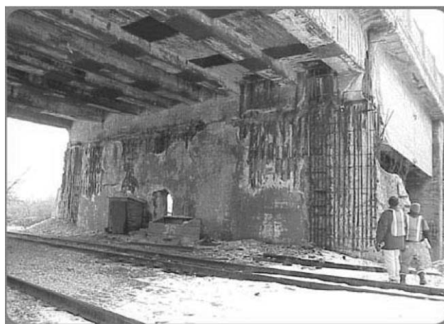
Fig. 4 The aging Rockefeller Road Bridge in Cleveland, Ohio, is one of many decaying bridges over the rail corridor. © Cuyahoga County Engineer's Office, Photo by Robert C. Klaiber, Jr., P.E., PS.; http://www.asce.org/reportcard/2005/assets/gallery/3-bridge.jpg .
