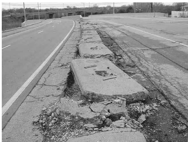
Fig. 2 Crumbling section of highway I-670, courtesy of the Ohio Department of Transportation (ODOT).
