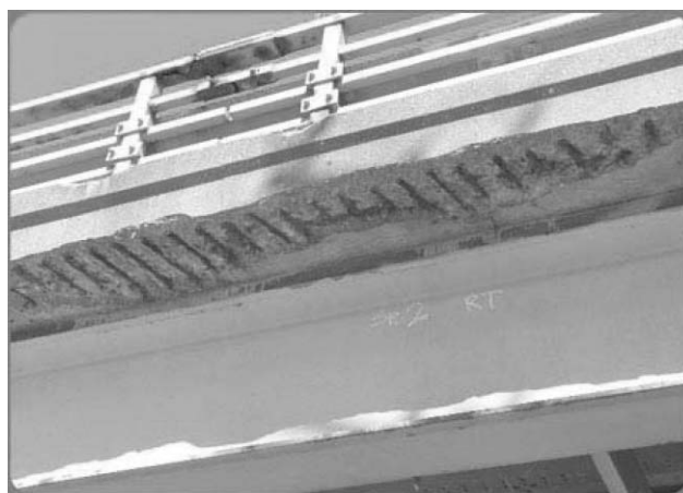
Fig. 5 As of 2003, 27.1% of the nation's bridges (160,570) were structurally deficient or functionally obsolete, an improvement from 28.5% in 2000. © Carl J. Lehman, Photo by Carl J. Lehman, P.E., F.ASCE; http://www.asce.org/reportcard/2005/assets/gallery/6-under.jpg .
